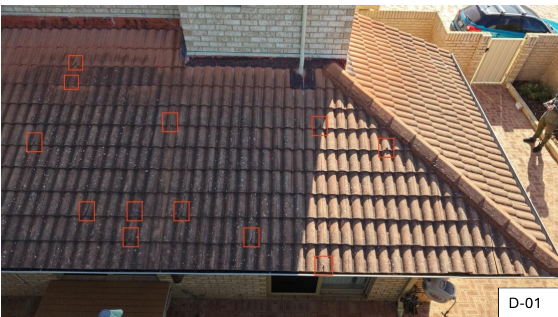
Image 1.2 – Localised tile chipping (D-01)
