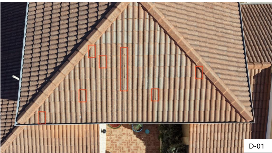
Image 1.6 – Localised tile chipping (D-01)
