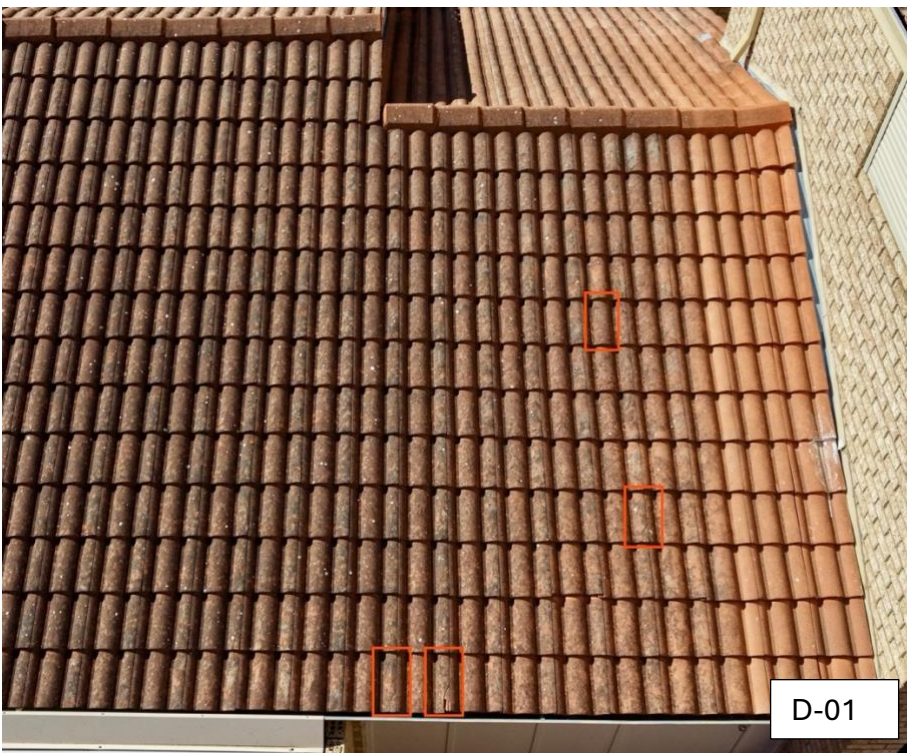
Image 1.4 – Localised tile chipping (D-01)
