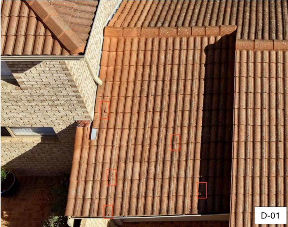
Image 1.5 – Localised tile chipping (D-01)
