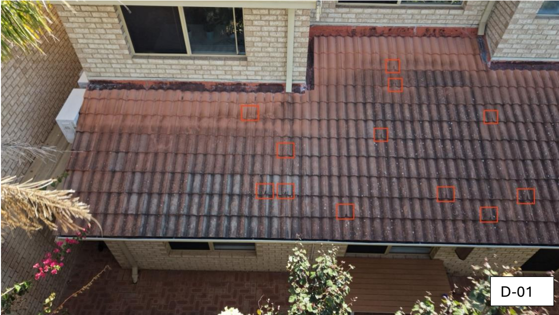
Image 1.3 – Localised tile chipping (D-01)
