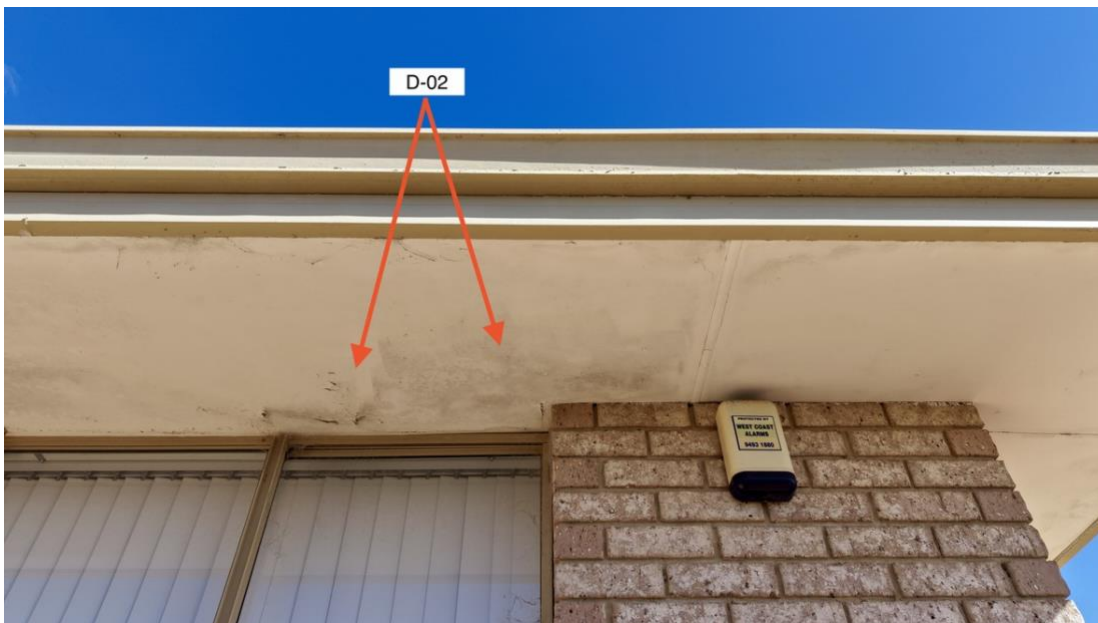
Image 2.2 – Water ingress – eaves (D-02)
