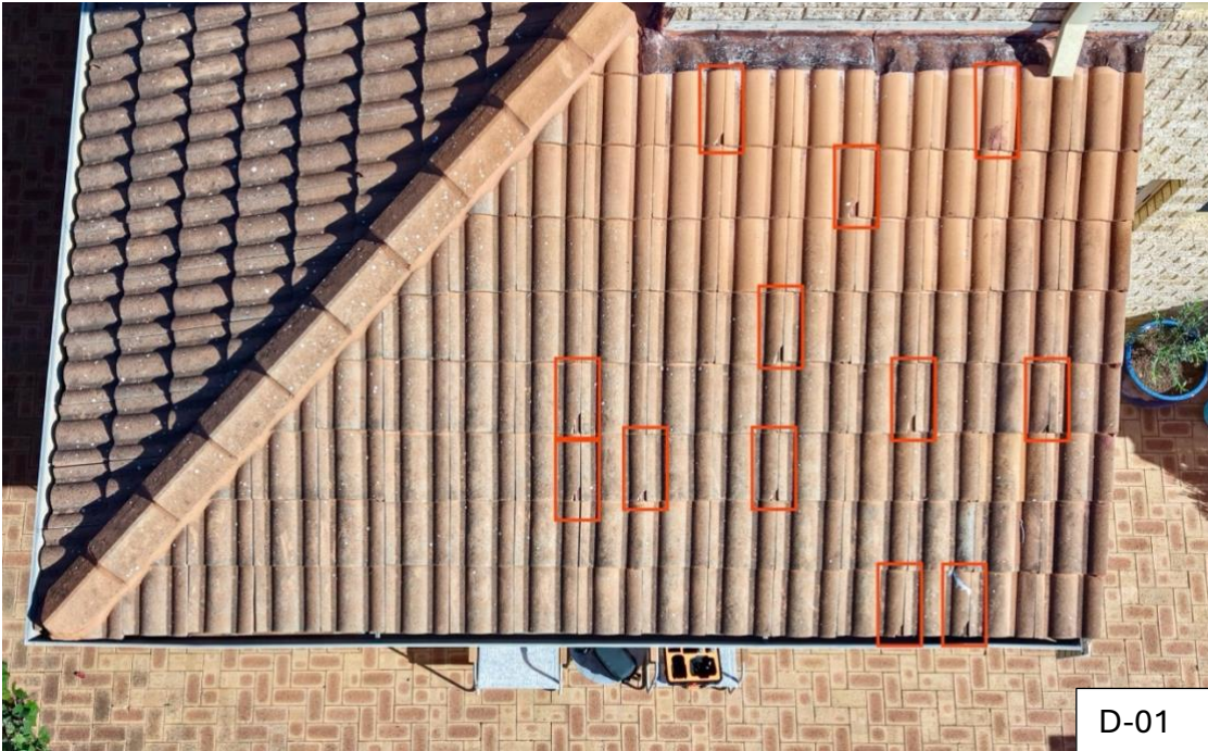
Image 1.1 – Localised tile chipping (D-01)
