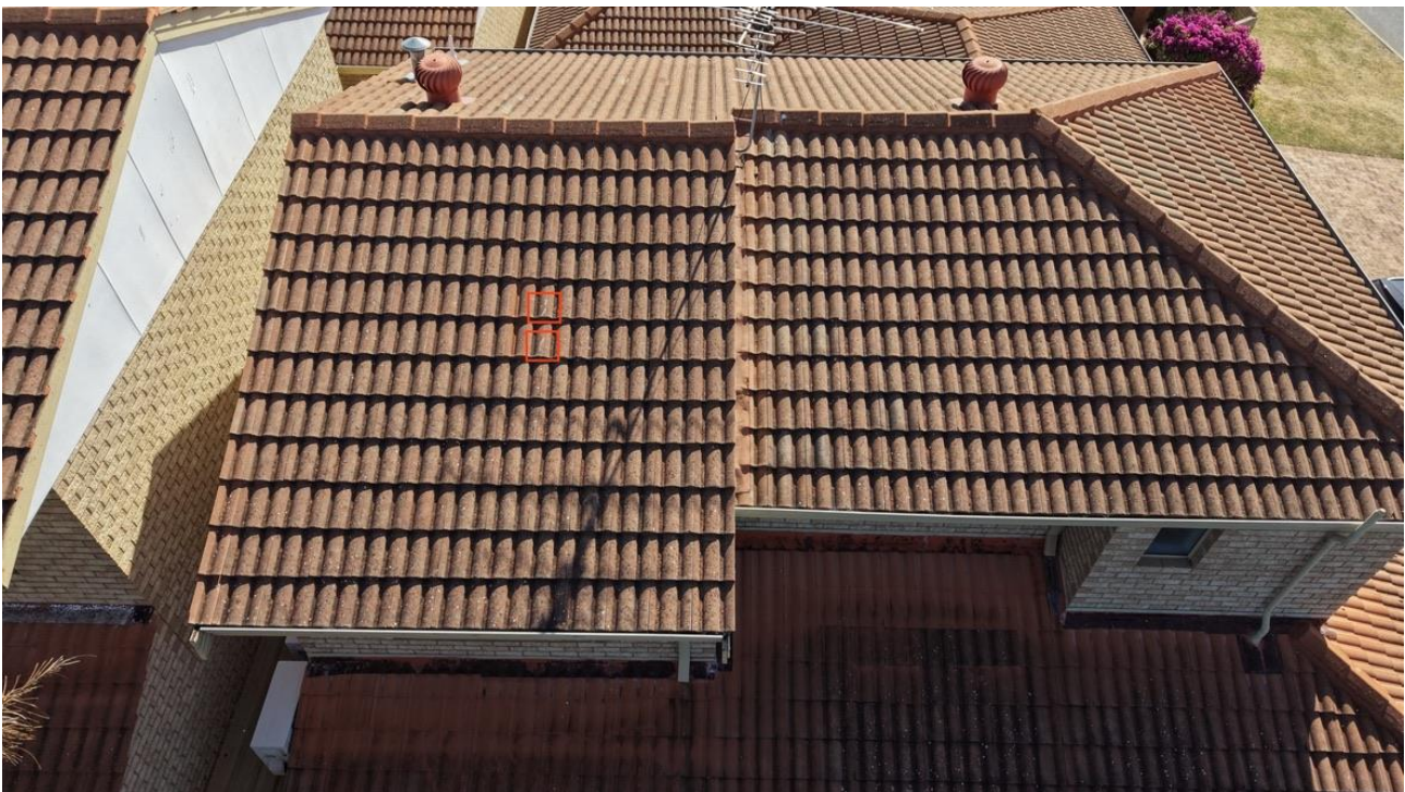
Image 1.8 – Localised tile chipping (D-01)
