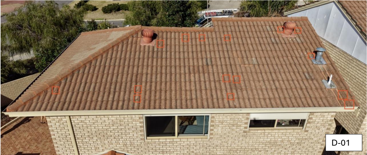
Image 1.7 – Localised tile chipping (D-01)
