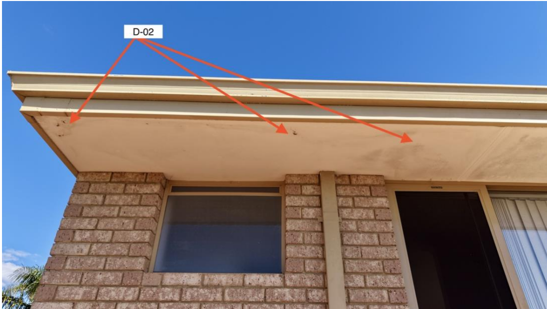
Image 2.1 – Water ingress – eaves (D-02)
